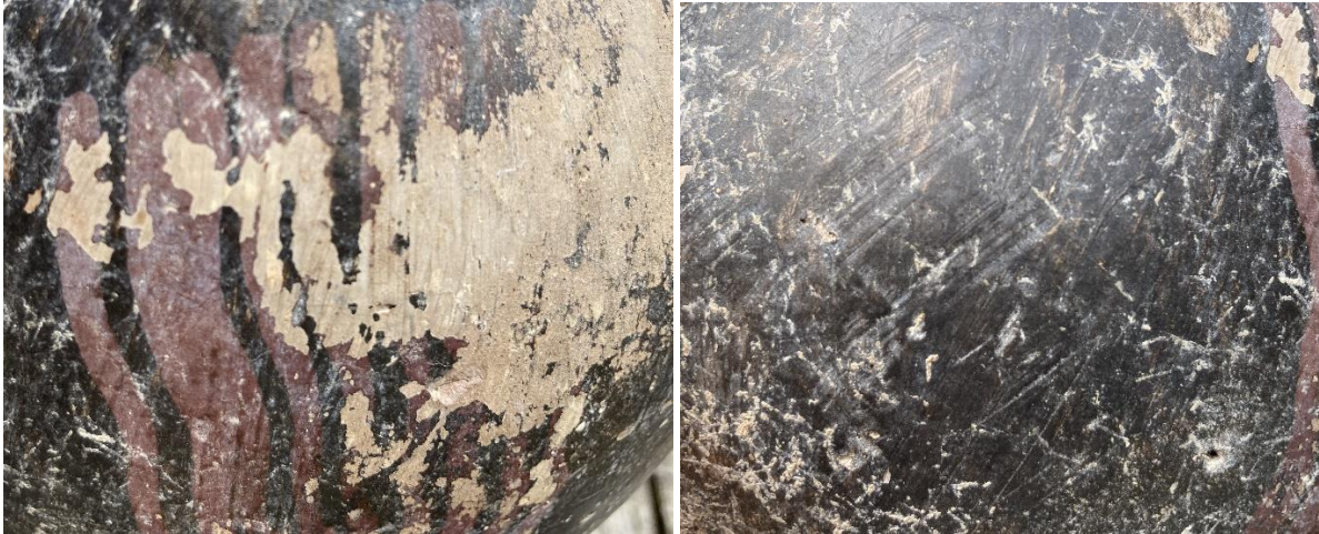
Slip flaking off
